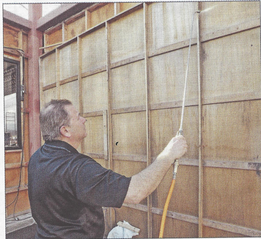
■ Randy Newman applies liquid Firetect with a sprayer to the back of a set facade on a sound stage at the Santa Clarita Studios lot. Photo by Dan Watson.
